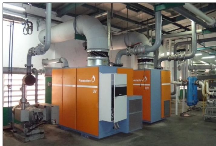
Centralized vacuum system for can production at Asia Packaging Industries in Vietnam
