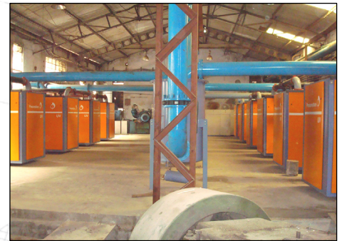
Pumps Room with 10 x UV50 VS90 HC
