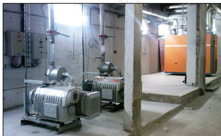
On left obsolete pumps, on right new UV30 VS55
