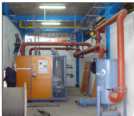
Pump room with 2 x UV30 from 2010
