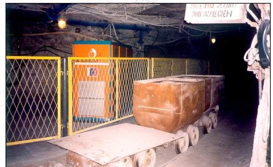
AS75/V air compressors in the Klodawa salt mine, 700 m below, running since 2002 @ 5,2 bar(g)
