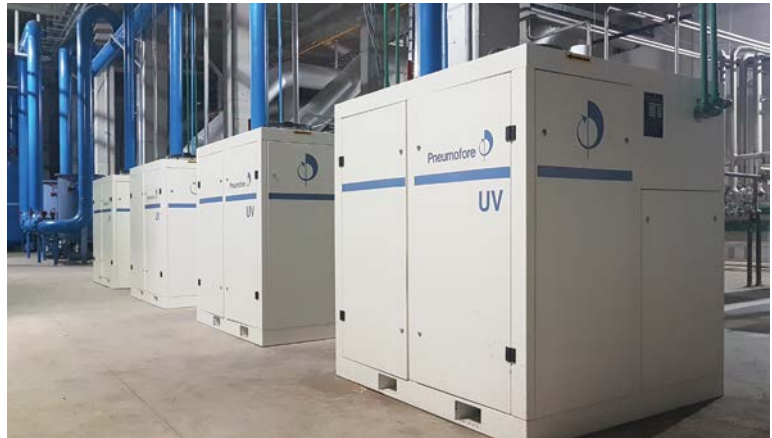
Pneumofore centralised vacuum system for glass manufacturing at Crown Vichisa, Mexico. Installed in 2017, the system comprises four units of UV24 VS45 rotary vane vacuum pumps.
